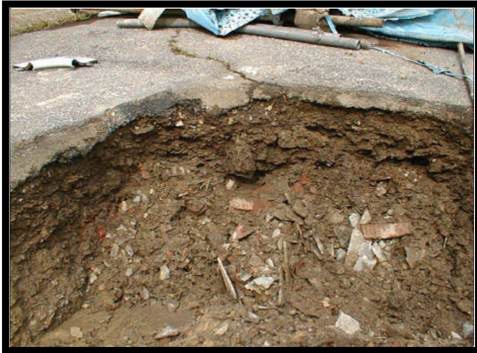
FIGURE 17. Plate scrap mixed with friable baghouse waste, used as fill beneath paved driveway.
