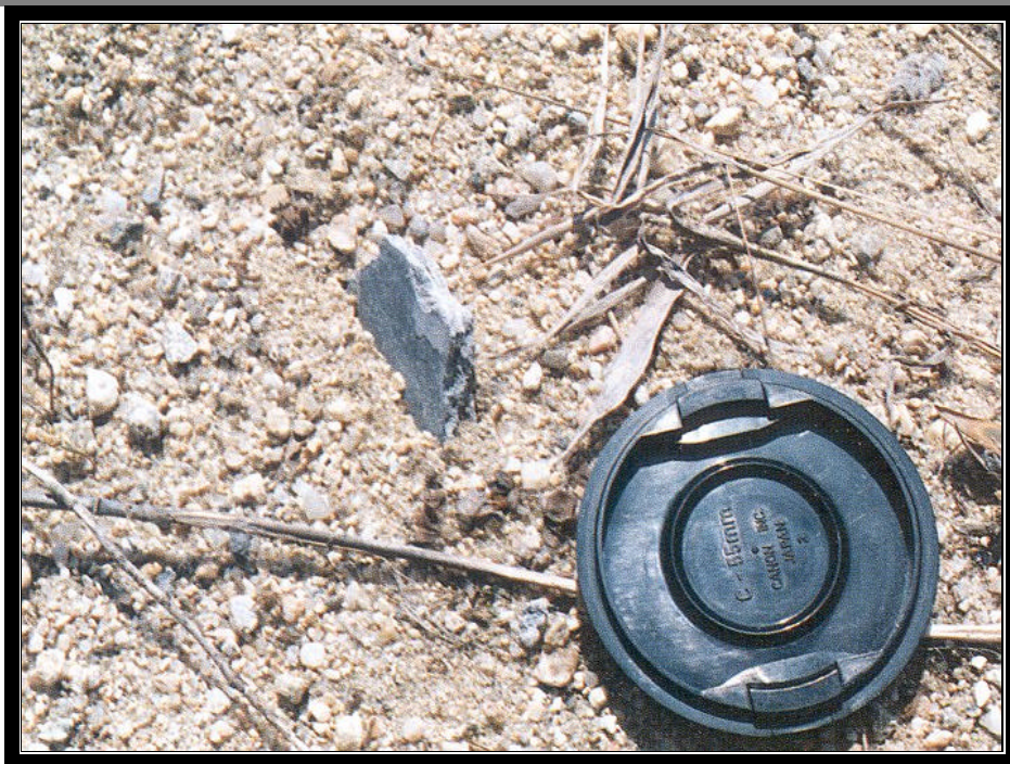
FIGURE 3. Protrusions of thin (1/4") irregularly shaped material from the soil may indicate that asbestos waste is buried below the surface. Round object in lower right is 2" diameter.
