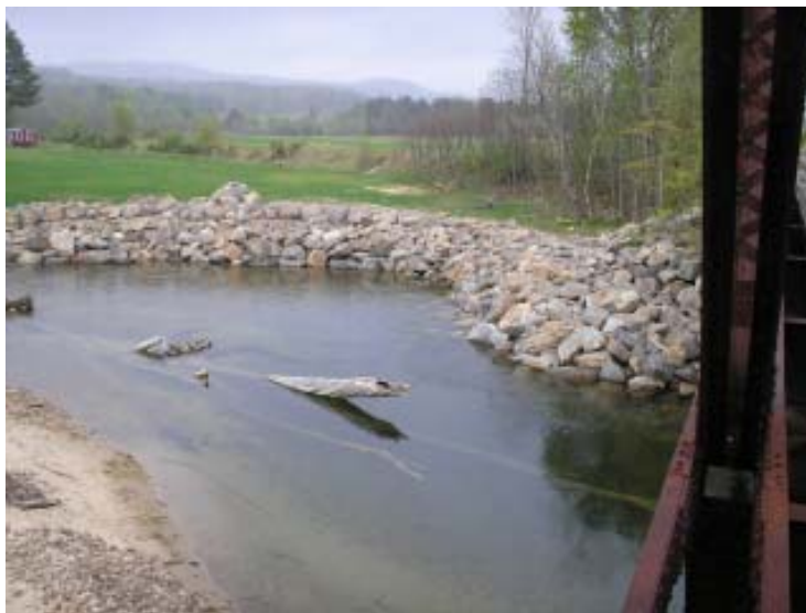
Figure 2-2: Photograph of an unnatural rigid design component on the Mad River in Compton, NH that was installed with minimal planning to fortify a rapidly eroding bank (Source: DES).
