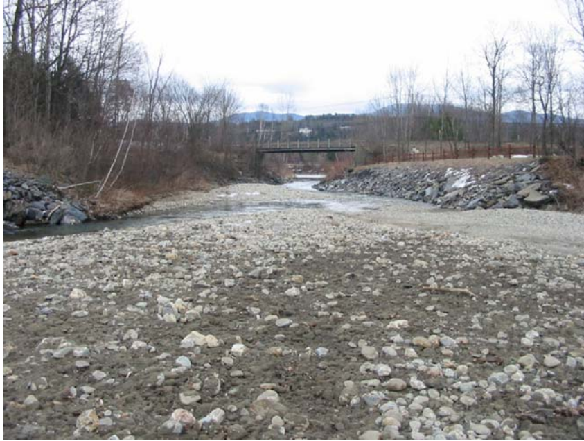
Figure 6-12: Excessive aggradation upstream of an undersized bridge on the West Branch of the Little River in Stowe, VT (Source: MMI). The photograph is taken looking downstream. The bridge opening is smaller than the current bankfull width of the channel. Hydraulic modeling indicates that backwatering takes place in this location under bankfull and larger storms.
