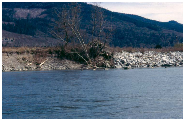
Figure 10-2: "Chasing the river" photograph where attempts to stop bank erosion with riprap lead to more erosion downstream on the Nooksack River, WA (Source: Field Geology Services).
