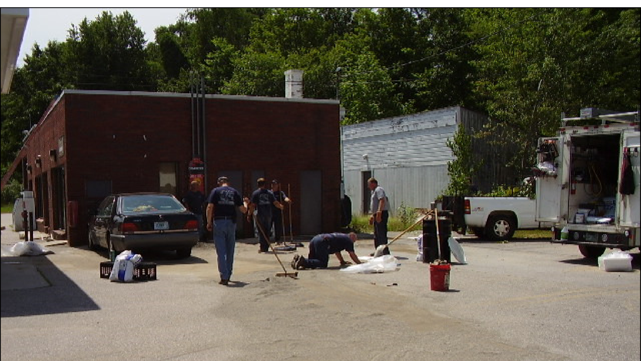
Overfill of Gasoline tanks during delivery
