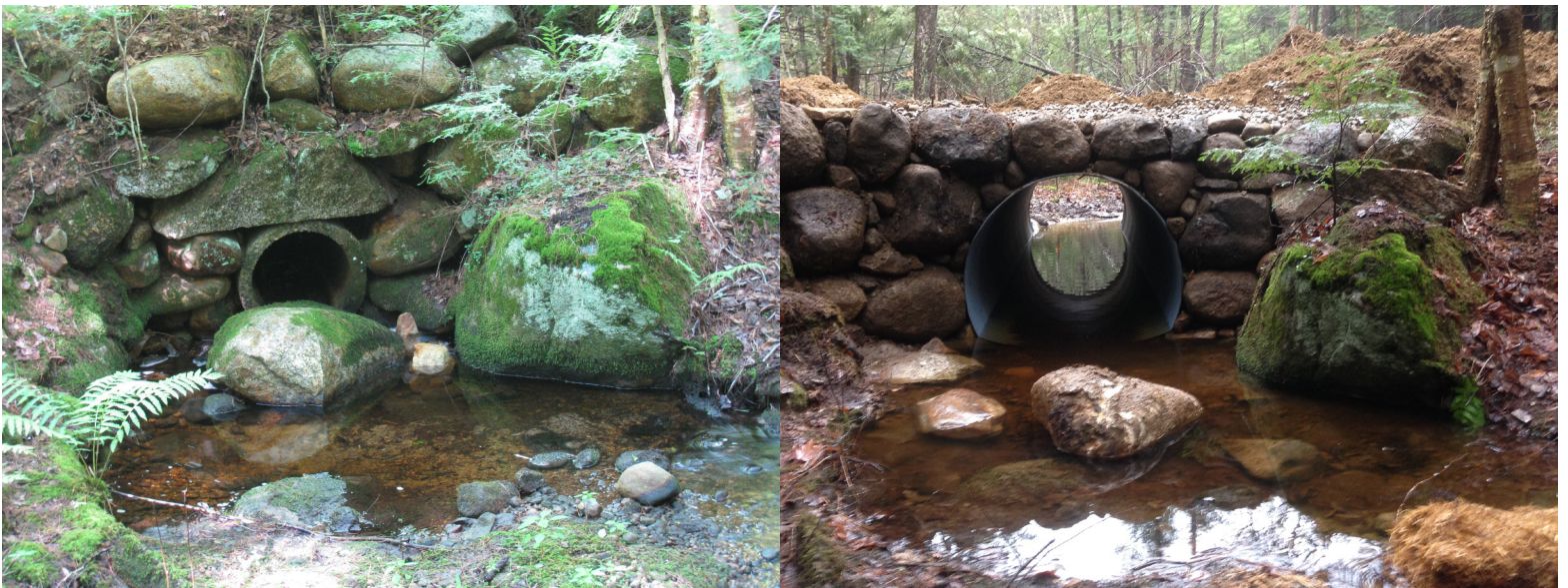
Avery Brook Woods Road culvert replacement project before and after – Frankestown, NH
