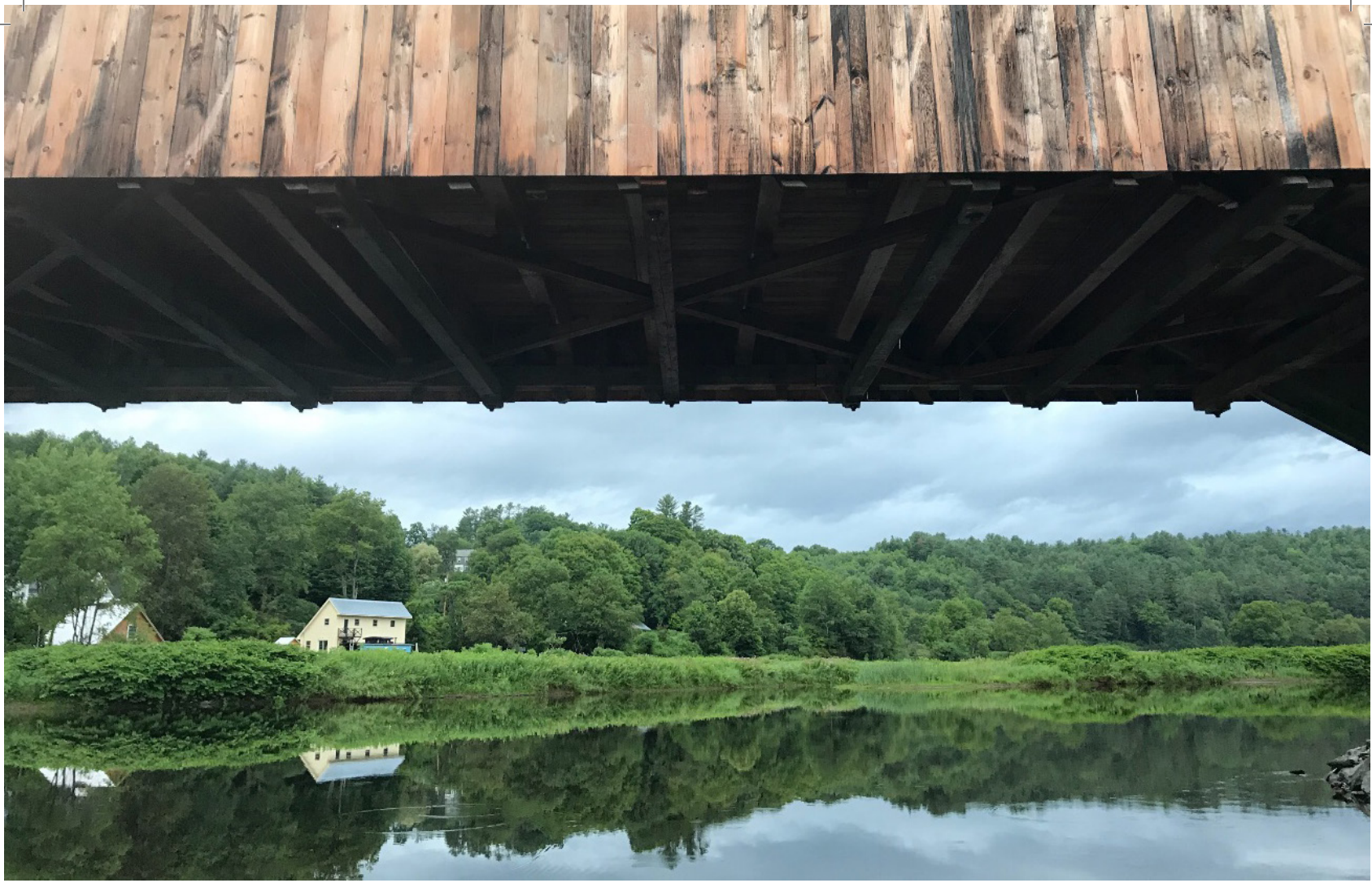
Pettyboro Road covered bridge over the Ammonoosuc River, Bath, NH – credit: Mary Ann Tilton
