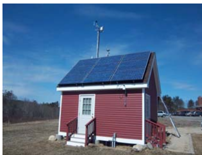
Multi-Pollutant Air Monitoring Station, Londonderry
